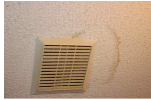
Old staining in Hall Bath exhaust fan
