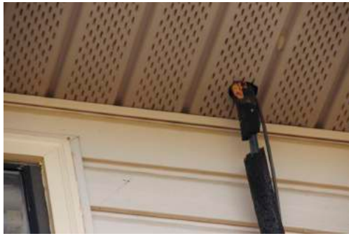
Closeup of refrigerant line
