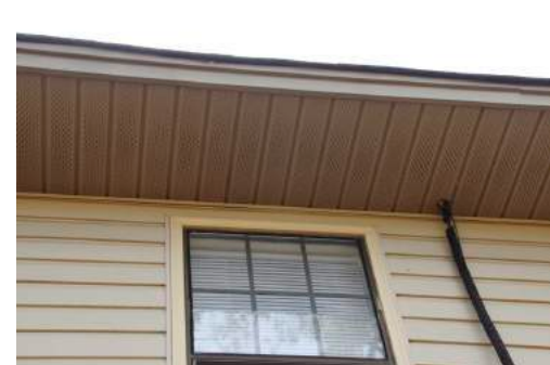
With insulated refrigerant through soffit
