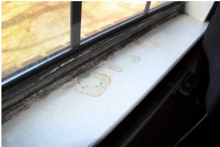
Master bedroom sill staining
