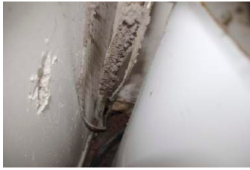
Left of water heater under AHU
