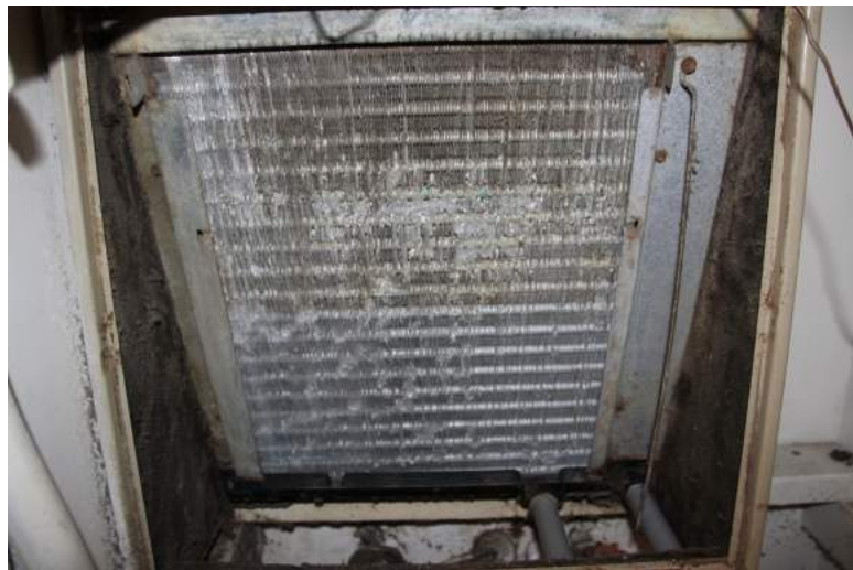
Damaged AHU coil
