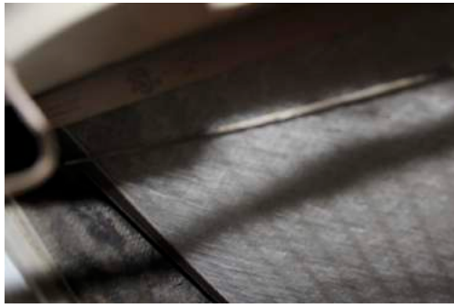
Left side, AHU interior
