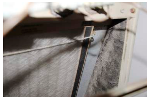
Right side, AHU interior
